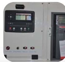
Control Panel & MCB
